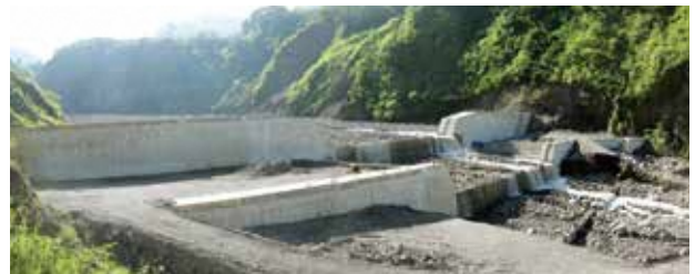
Indonesia : Sabo Dam in Jeneberang River (Courtesy of Yachiyo Engineering Co., Ltd.)
