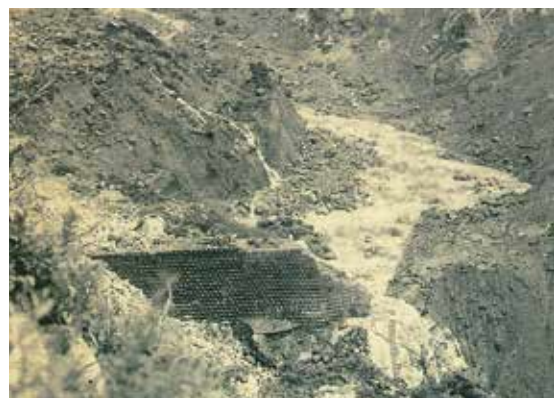
Yukawa No.1 Sabo Dam broken by debris flows
